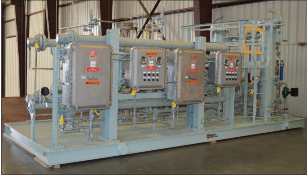
Redundant NEMA 7 panels for un-manned compressor station
